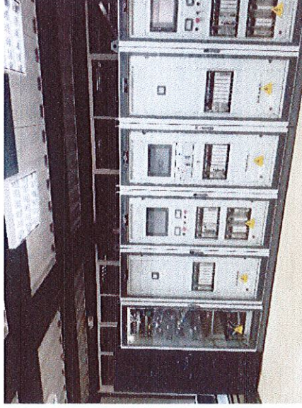
Figure 11: PLC de Casa Maquina
